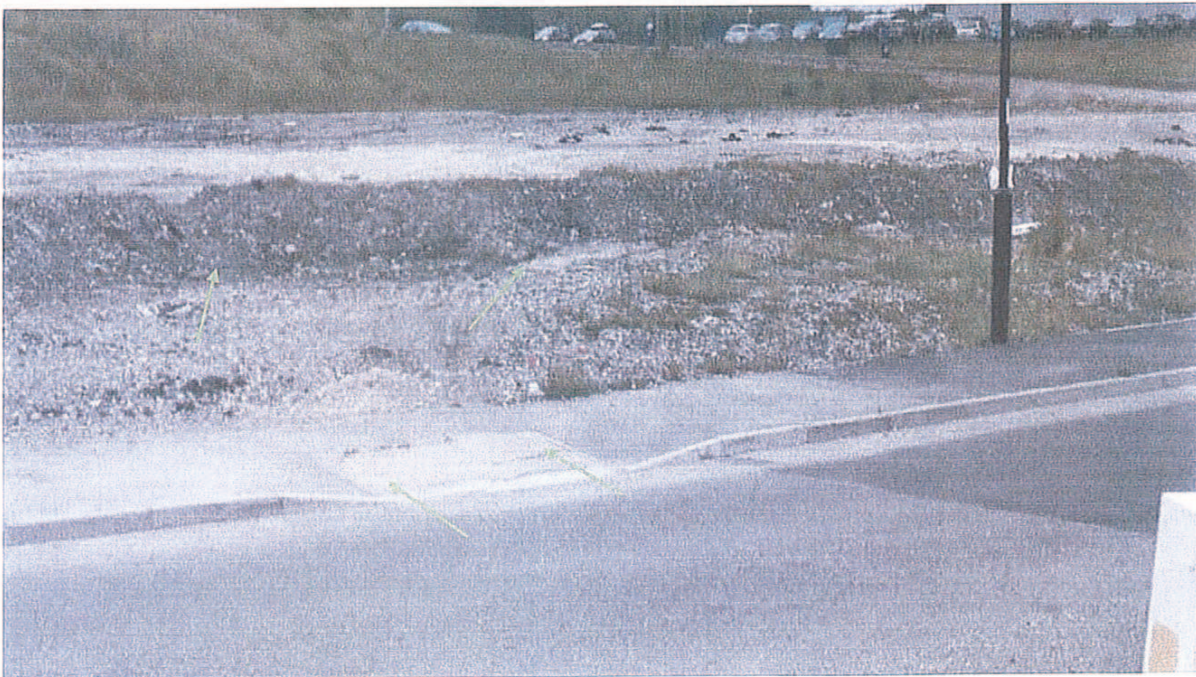
Plate 8a Shallow bunds low enough to drive over on Cowley Way. Dropped kerb allowing easy access for vehicles.
