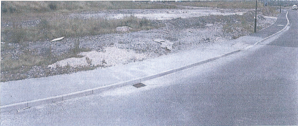
Plate 8 Shallow and incomplete soil bunds on Cowley Way. Dropped kerb allowing easy access.
